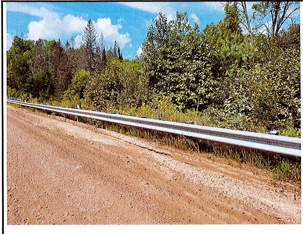
Photo 7 Accumulation of dirt below approach guide rail
