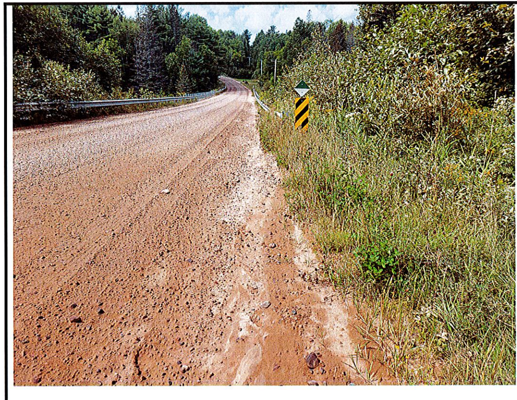
Photo 8 Vegetation overgrowing approach guide rail
