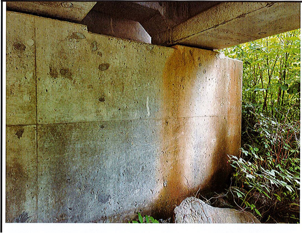
Photo 13 Damp staining and rust staining on east abutment wall
