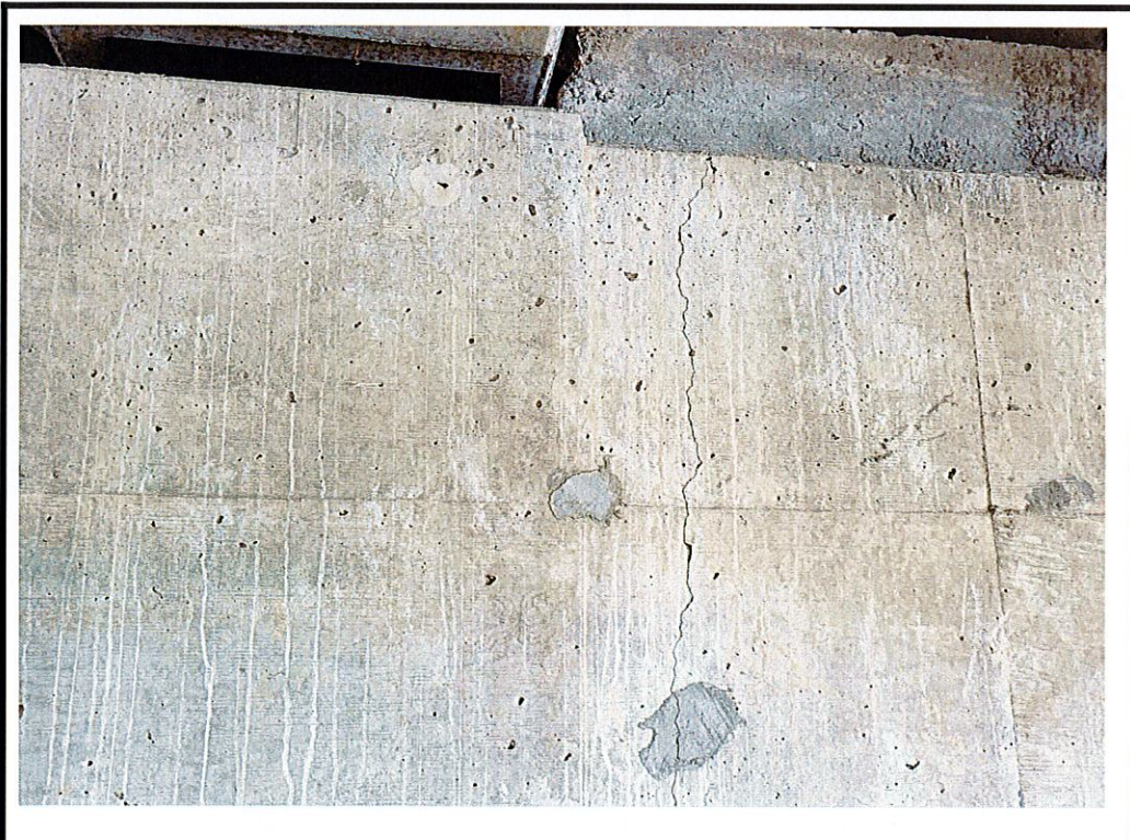
Photo 14 Narrow vertical crack on abutment wall
