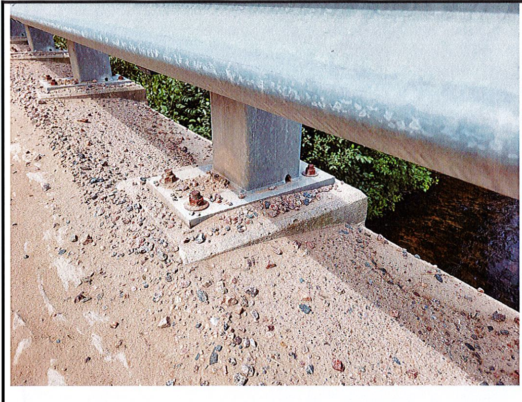
Photo 9 Light corrosion of anchor bolts on deck post base-plates
