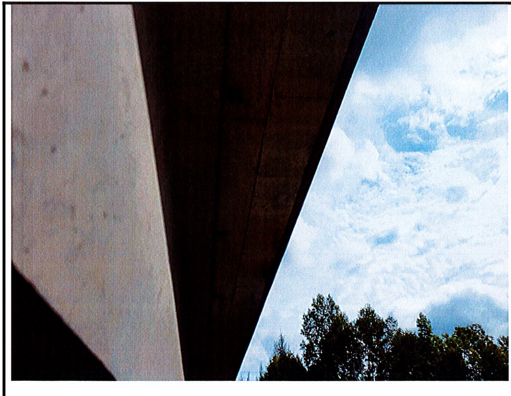
Photo 12 Isolated small spalls and rust staining on exterior soffit
