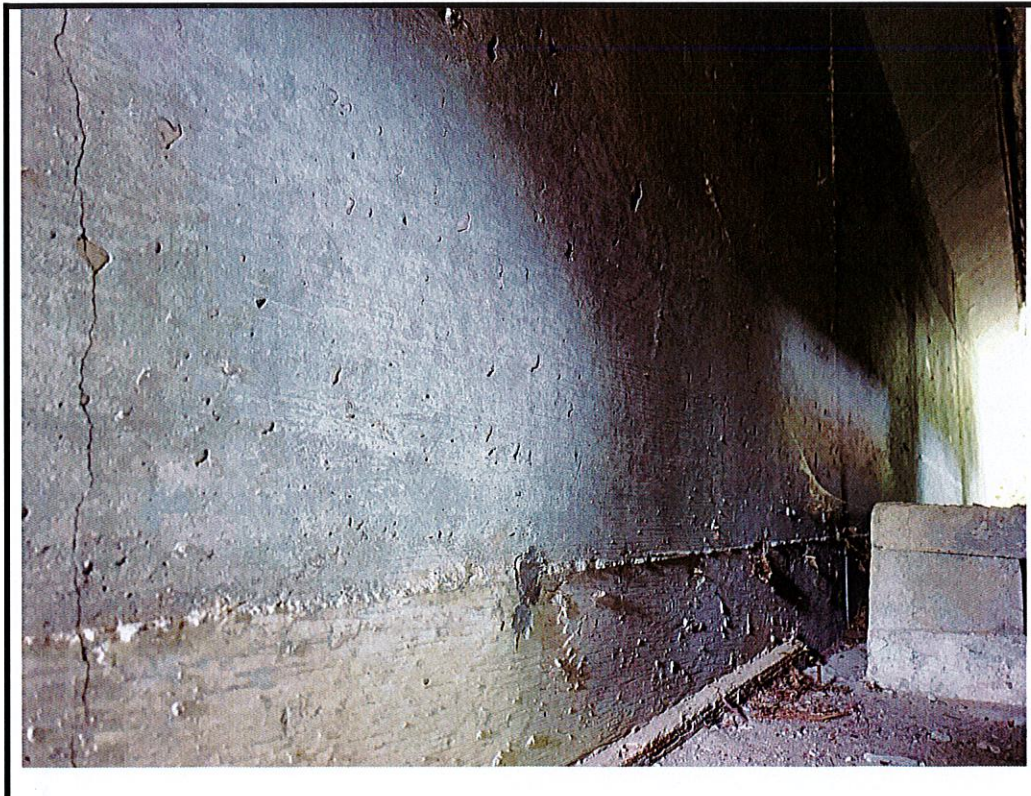
Photo 10 Narrow vertical crack on east ballast wall
